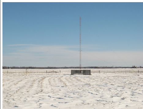
One of 3 antennas at CHU
