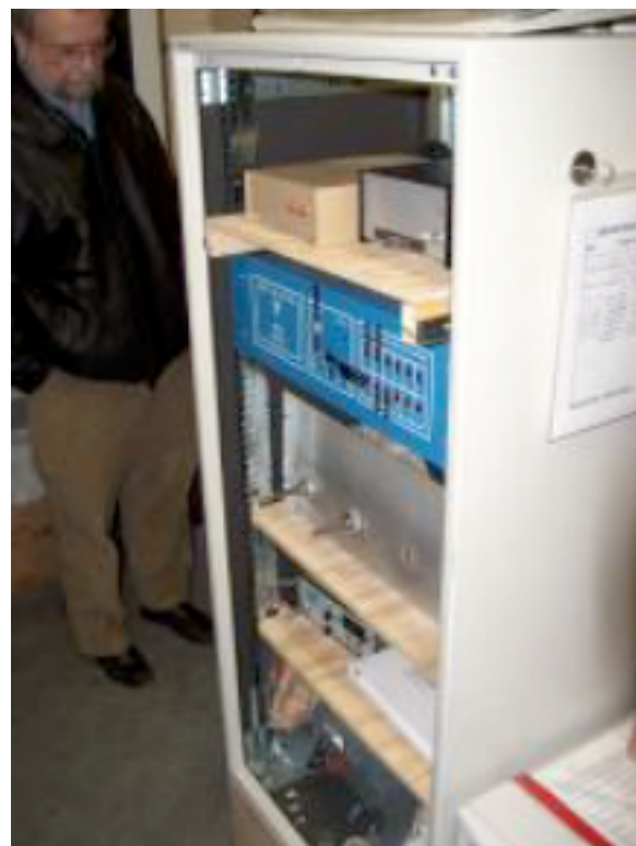
repeater rack-- greatly improved
