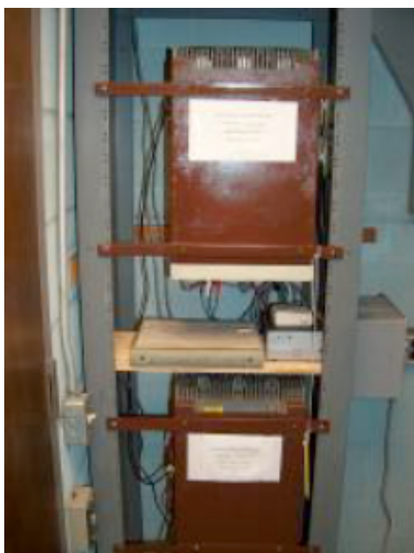
battery back up
